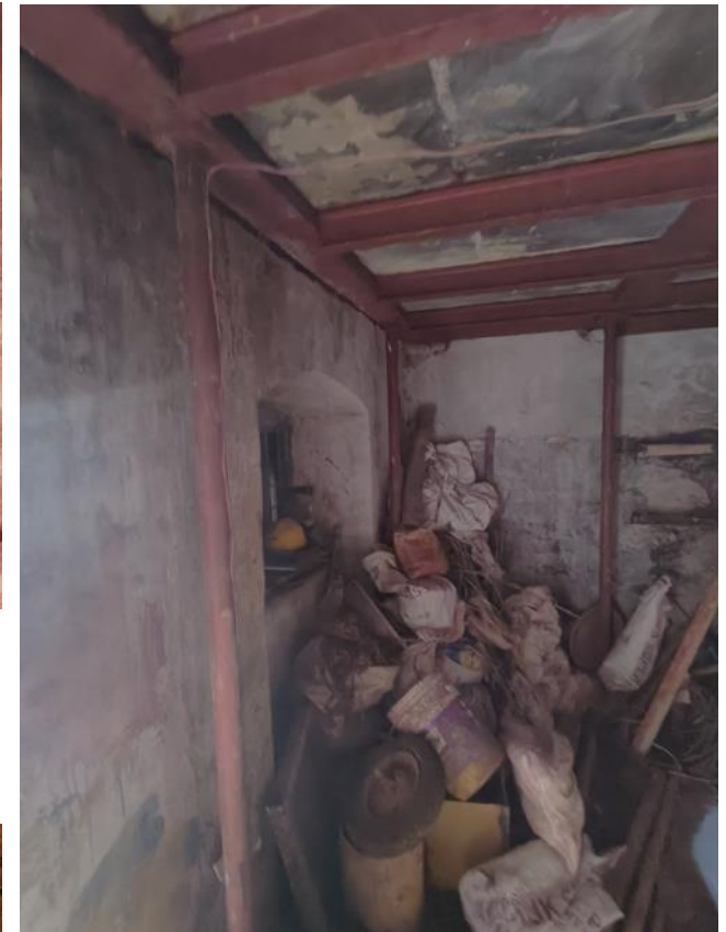
Removing the Mild steel structure in the store rooms below the kitchen block and structurally casting a new RCC slab
