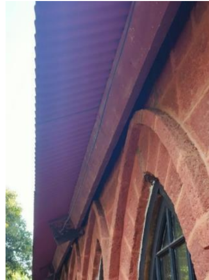
Remove damaged/ warped wooden roofing structure member with new Mild steel structure as this room has wooden ceiling.
