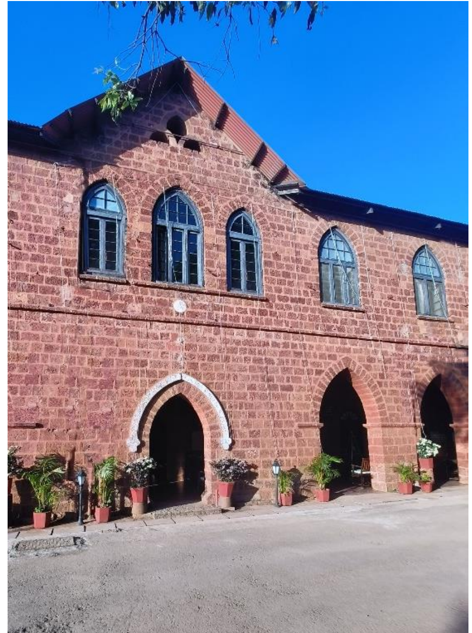
Removing existing stone ware & GI pipes on the front facade by re-routing them through the internal passage.
