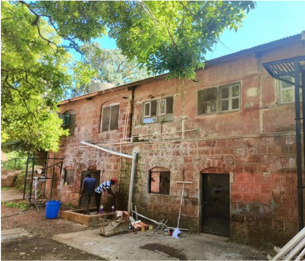
Removing brick wall & wooden posts and introducing laterite wall to support the existing roof of kitchen
