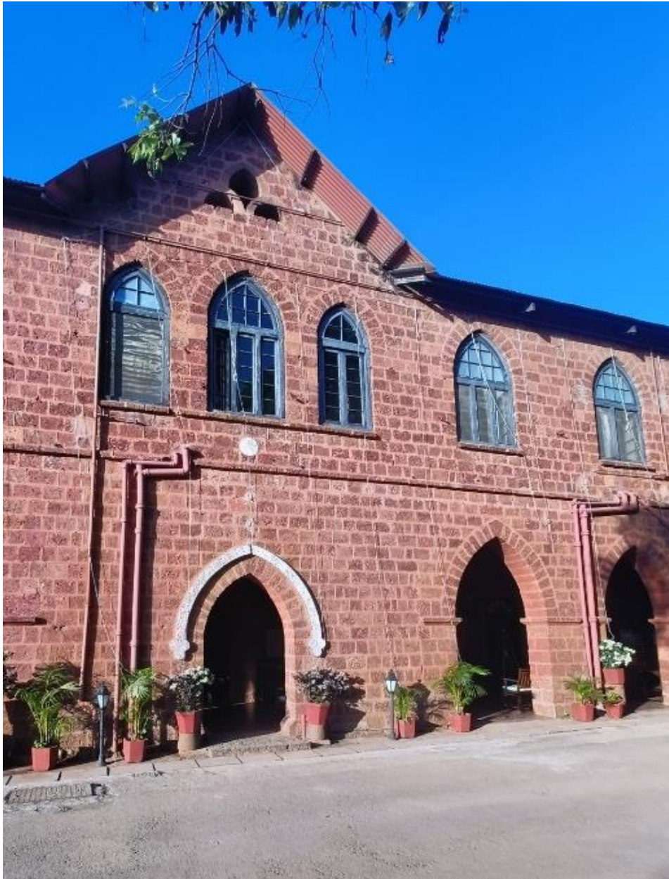
Note the existing stone ware and GI pipes on the main facade
